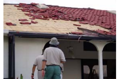
Exposed Sheathing and Tile Damage
