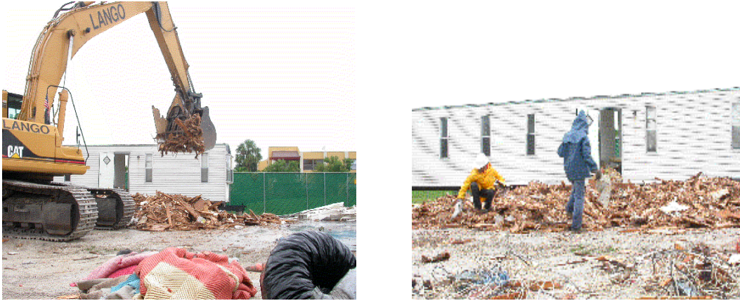
Figure 18. (Left) Backhoe forming a pile of wood. (Right) Collection of recyclable materials from wood debris.
