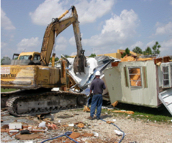
Figure 10. Backhoe in the process of shearing off the exterior aluminum sheets from the walls of a mobile home.
