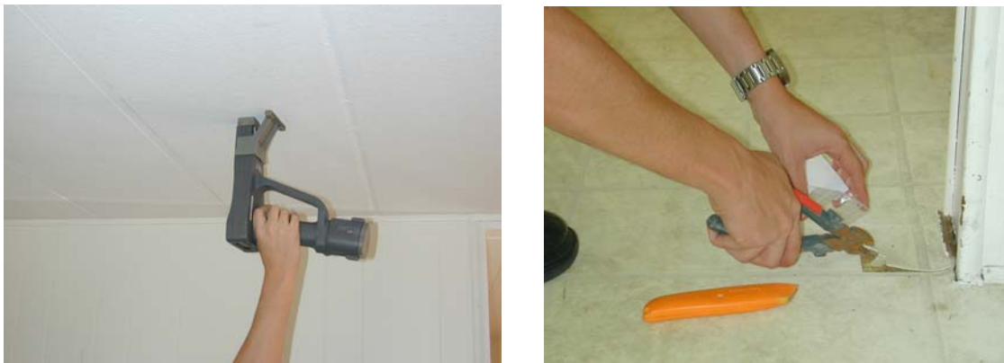
Figure 9. Lead and asbestos inspection of a double-wide mobile home unit at Davie, Florida.
