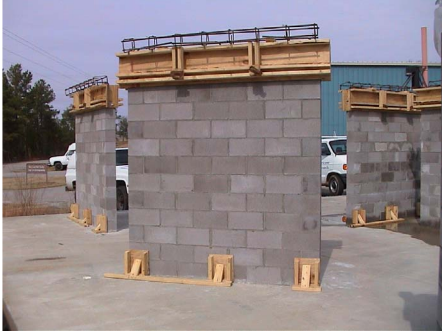
Figure 4. Reinforcing Cage and Formwork for Casting Reinforced Concrete Tie Beams for HVHZ Walls.
