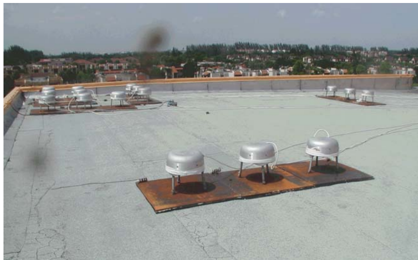
Figure 7. Pressure Sensors Installed on the Roof
