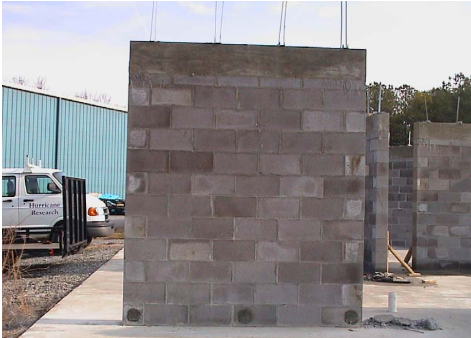
Figure 8. NU VUE Industries NVHTA 20 Hurricane Straps in Finished Reinforced Concrete Tie Beam Wall.
