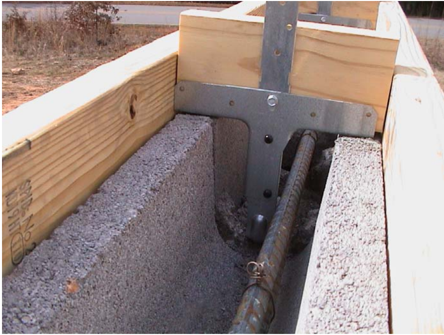
Figure 6. Simpson Strong-Tie HETAL 20 Placement in CMU Bond Beam Before Grouting of Bond Beam.
