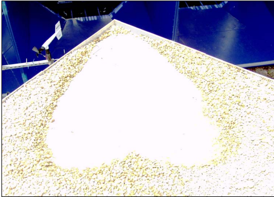
Figure 32. Gravel Scour Associated with Drain-Thru Gravel Stop
