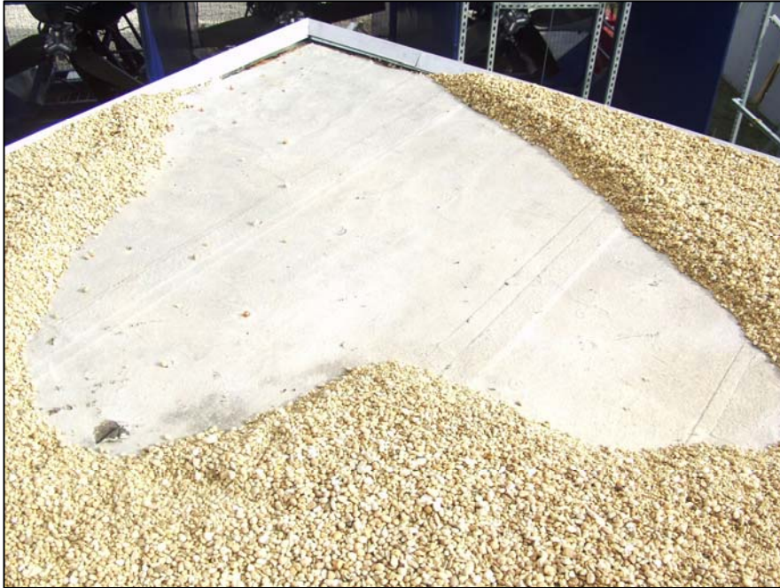
Figure 35. Gravel Scour Associated with Econosnap Fascia at 4400 rpm
