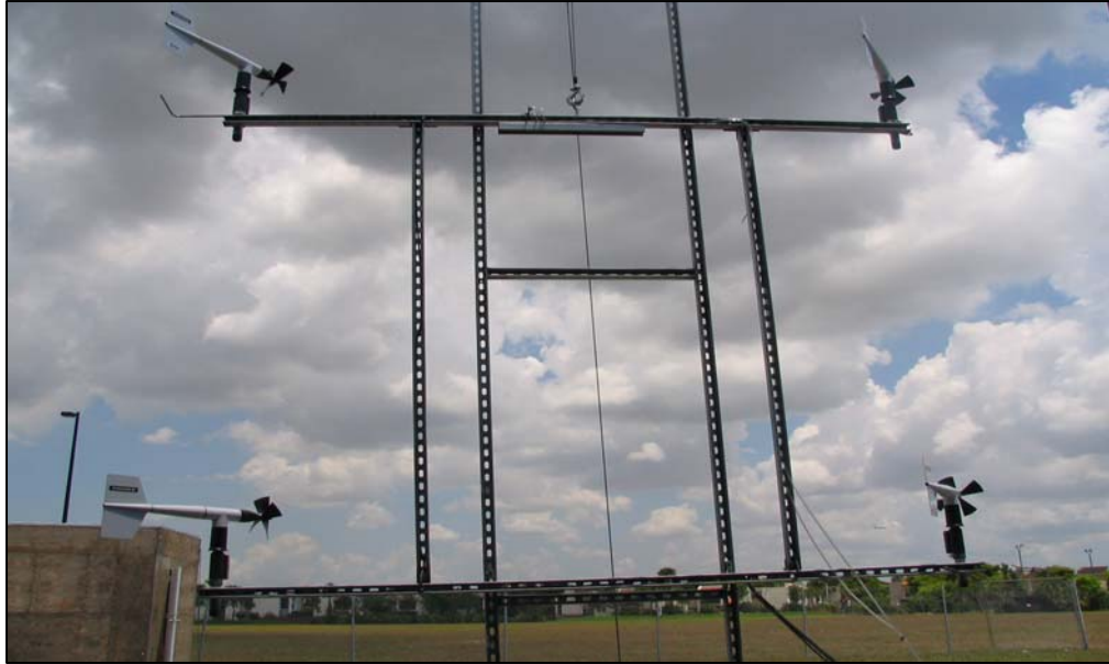
Figure 18. Close-up of Wind Monitor Frame Equipped with Four Wind Monitors
