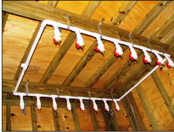
Figure 9. PVC Reference Pressure Manifold
