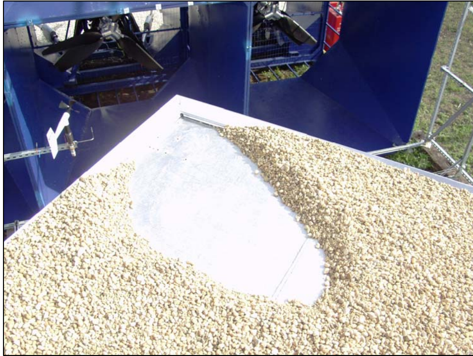
Figure 31. Gravel Scour Associated with the Econosnap Edge Fascia
