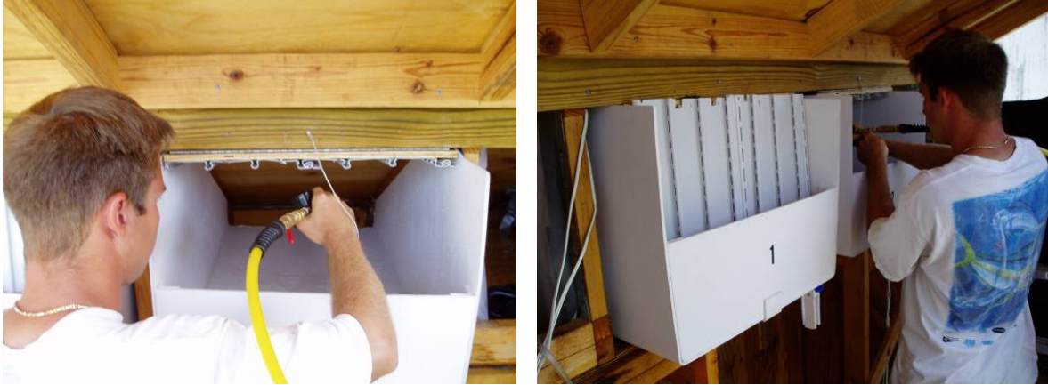
Figure 16 Collection of Water in Catch Basins
