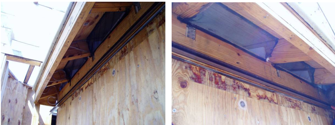
Figure 10 Use of Insect Screen to Retard Wind-Driven Intrusion into the Attic Space
